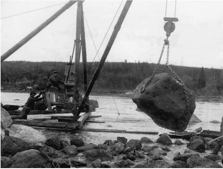
Figure 4. Motorized crane clearing the stream channel and building a stone pier in the Ume River (1930s). Photograph courtesy of Västerbotten's Museum, Umeå.
